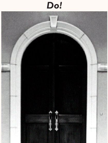
Forethought and attention to detail would have eliminated that short piece just below the arch on this otherwise graceful door surround.
